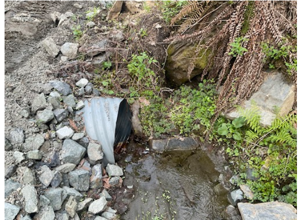
Upper culvert inlet partial plug
